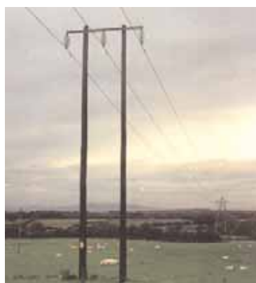
Typical (38kV) line. Requires wayleave and planning permission.
