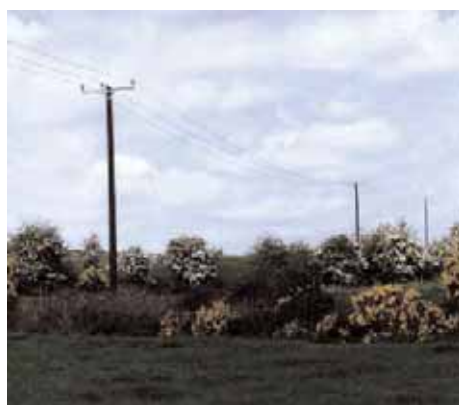
Typical Medium Voltage (10kV or 20kV) line. Wayleave clearance required but not planning permission, except in particular circumstances.
